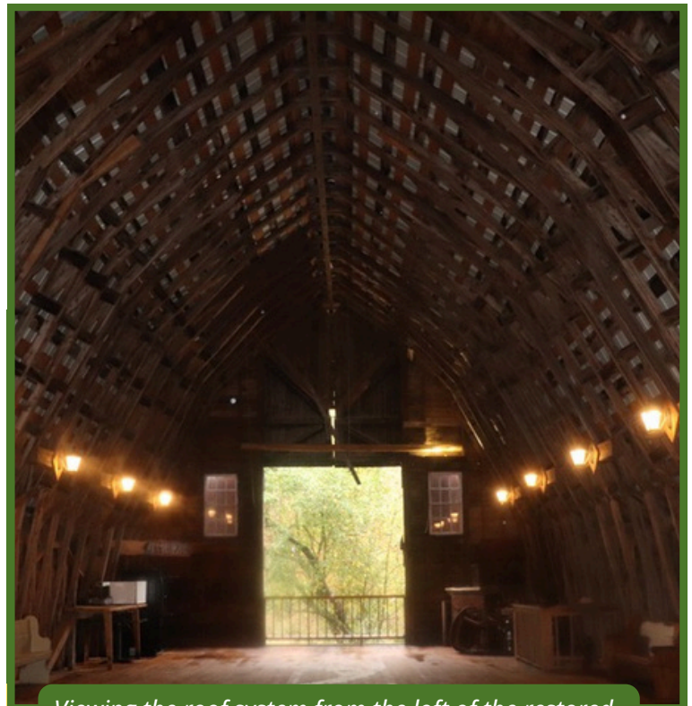
Viewing the roof system from the loft of the restored gambrel barn, which was once an event space.
